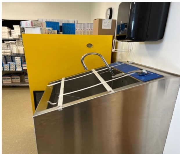
Figure 4: Out of service scrub sink in clinical area. Sinks and other areas of limited use pose a risk for stagnation.
