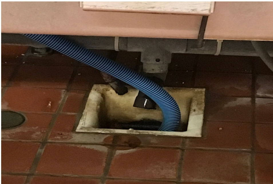
Figure 3: Improperly installed drain line. Drain line must be at least 3 inches above drain to prevent backflow into systems.
