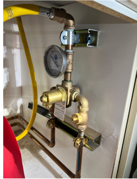
Figure 8: Mixing valve under sink.
