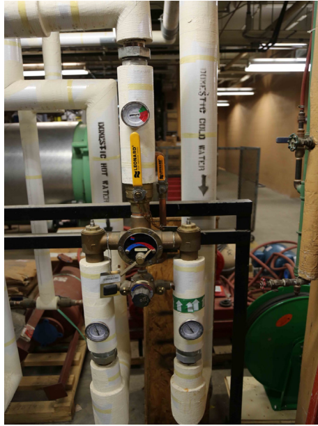
Figure 7: Mixing valve in a mechanical space.
