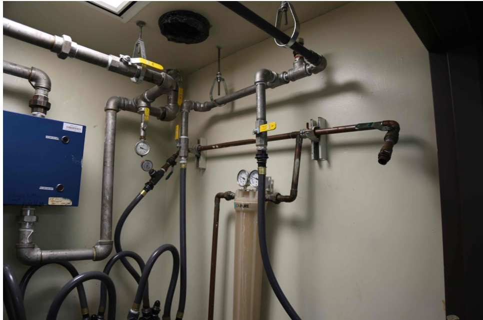
Figure 6: Dead end piping from abandoned system.
