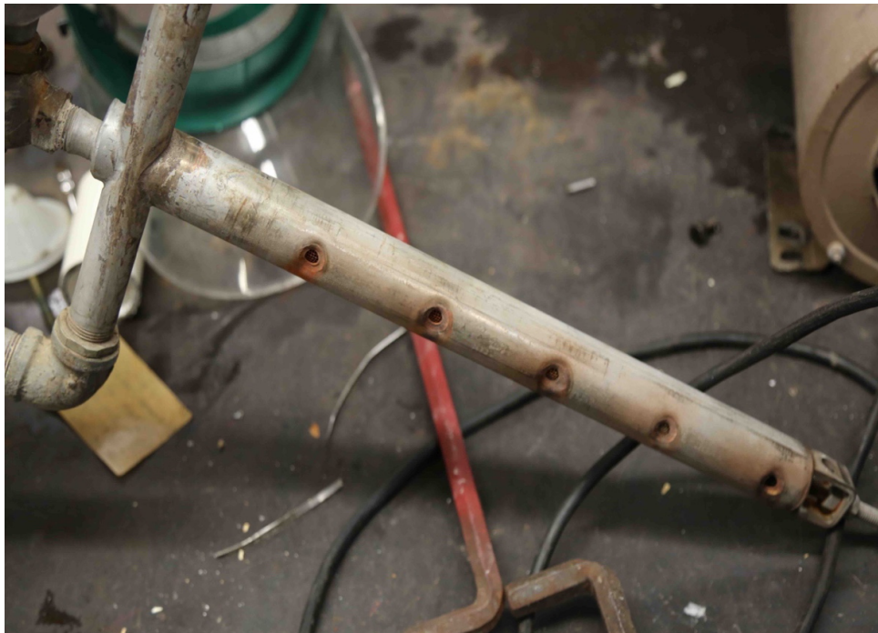
Figure 5: Lack of maintenance on a humidifier.
